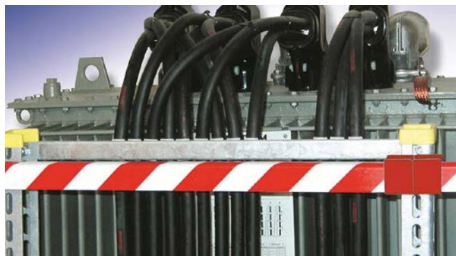
Barrier in a transformer station.
