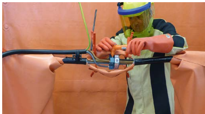
Covering live parts.
